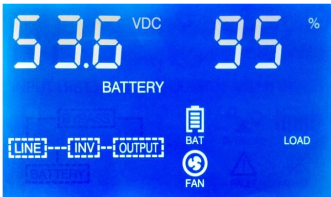
显示电池输入电压53.6Vdc
